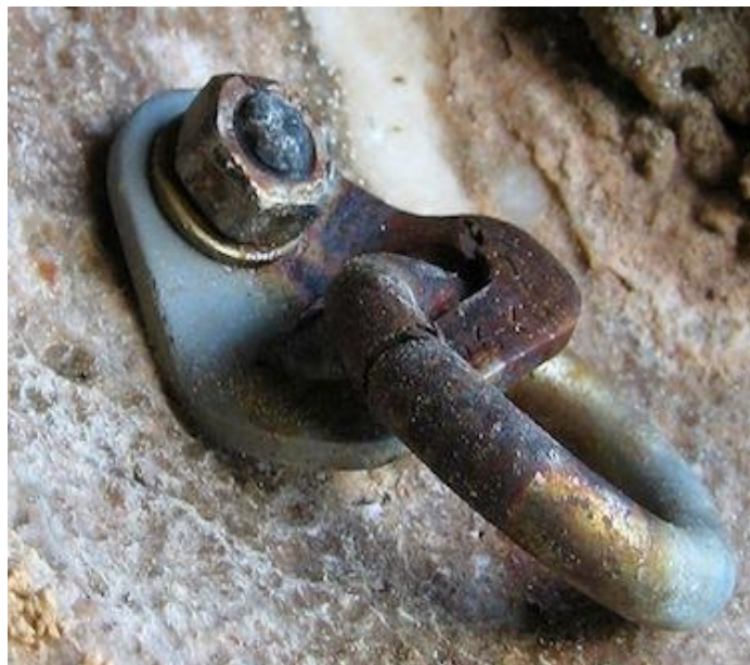
A severely corroded stainless steel bolt and hanger. If it hasn't fallen off yet, you can see this bolt in the cave on "Shooting the Curl" at the Wave Wall. Obviously, don't even think about clipping this or lowering off it! Hamilton
