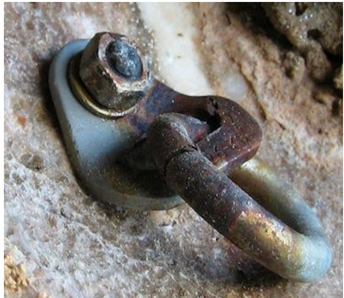
A severely corroded stainless steel bolt and hanger. If it hasn't fallen off yet, you can see this bolt in the cave on "Shooting the Curl" at the Wave Wall. Obviously, don't even think about clipping this or lowering off it! Hamilton
